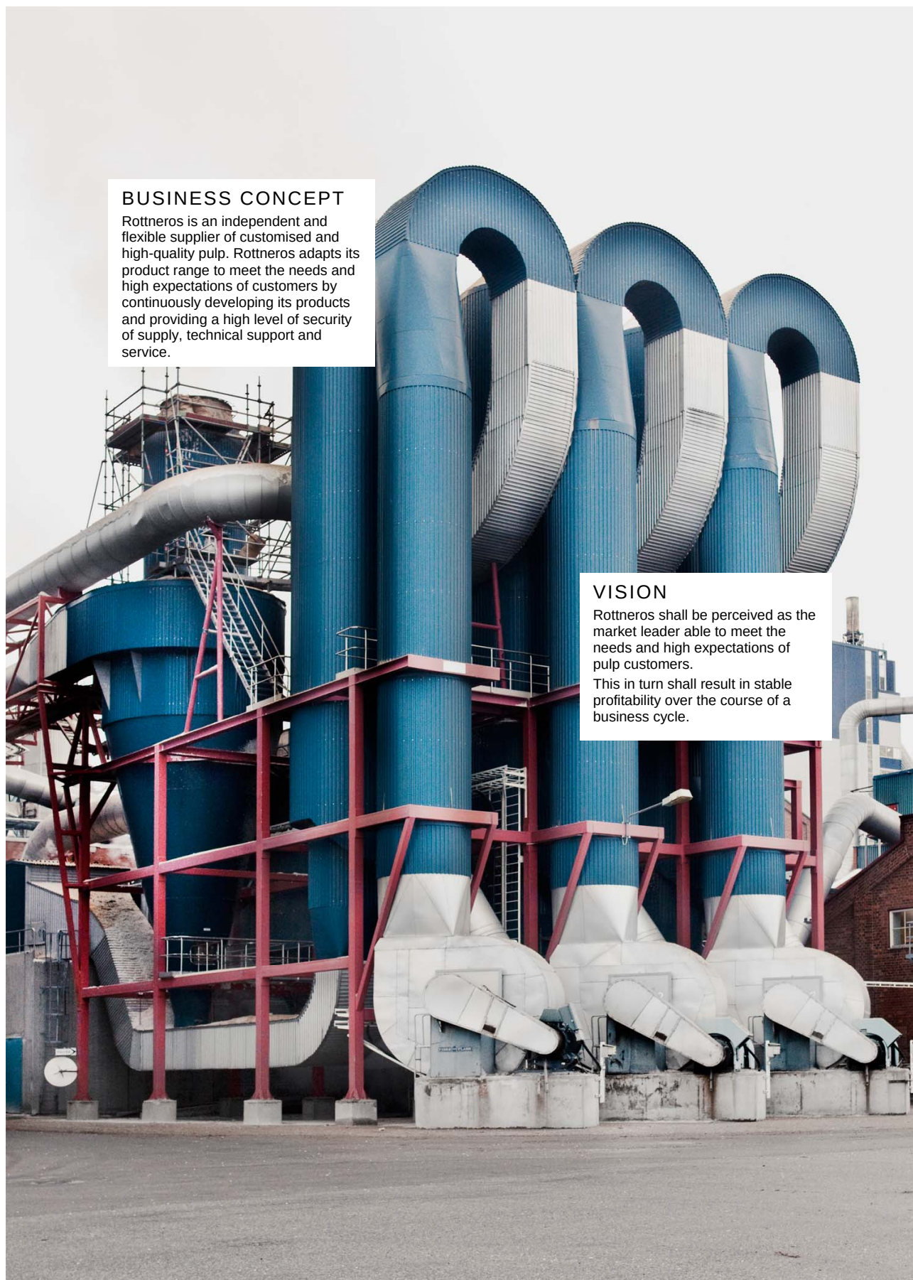
Flash drying at Vallvik Mill. This kind of drying is one of the prerequisites for the specialist pulps produced at the mill.
